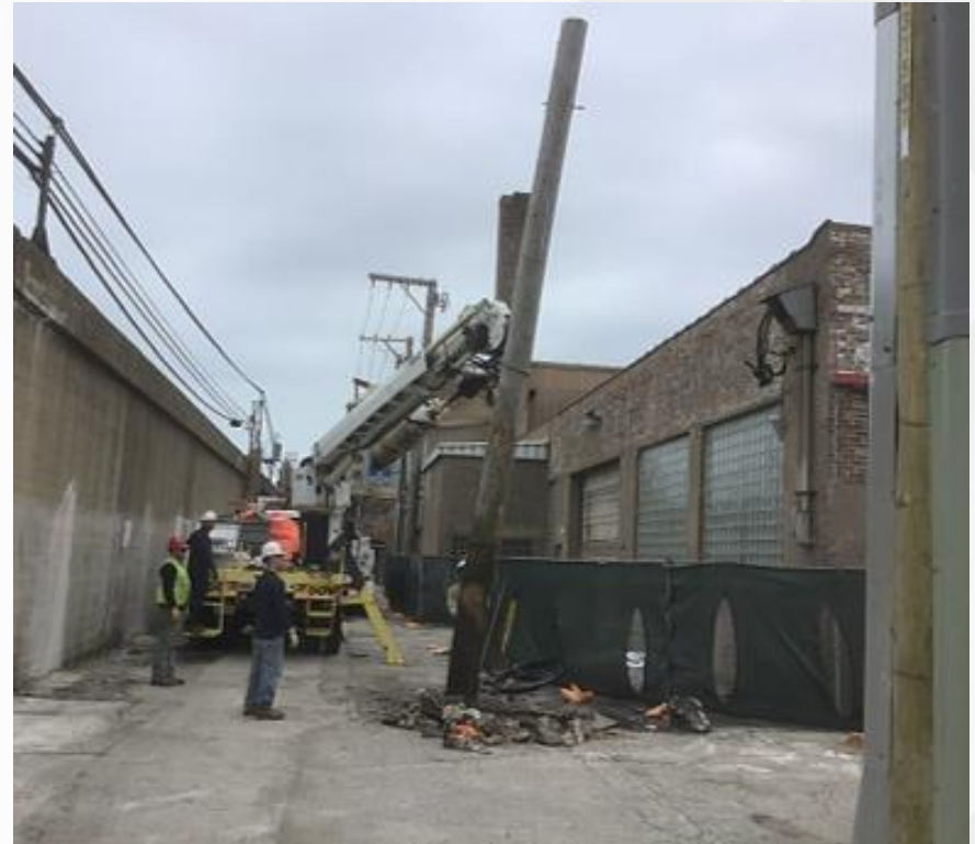
Removal of a utility pole near Bryn Mawr as part of the RPM Phase One Project, 2019
