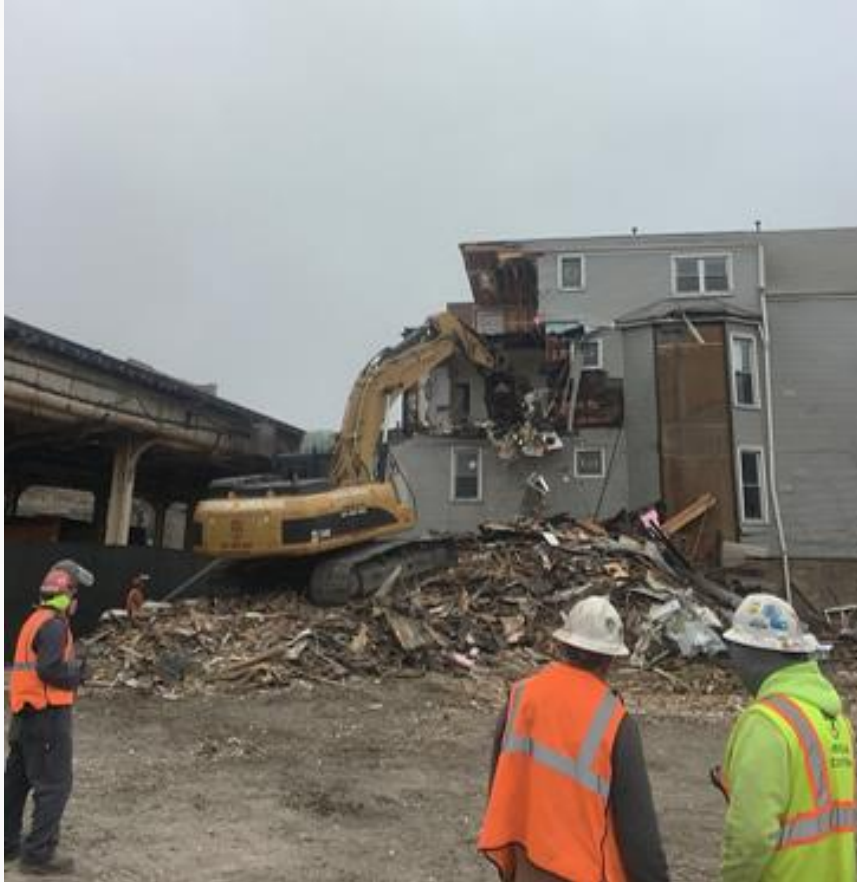
Property demolition for the Red and Purple Modernization (Phase One) Project north of Belmont, 2018
