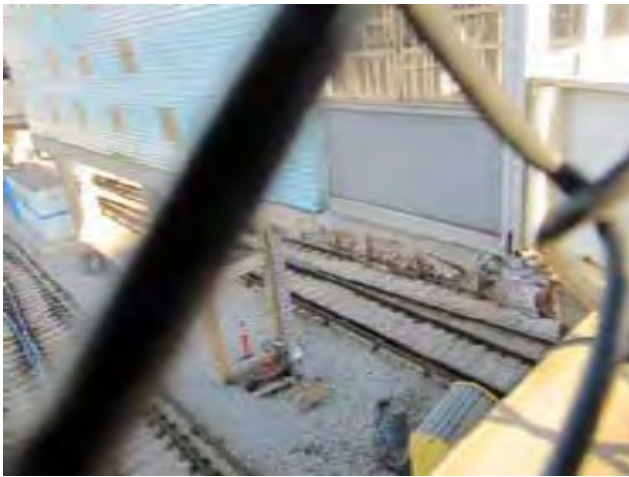
View extensive concrete deterioration and spalling at Loomis stationhouse
