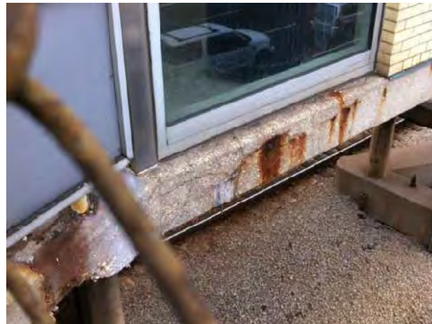
View of corrosion and rusting at concrete at base of Morgan stationhouse walls.
