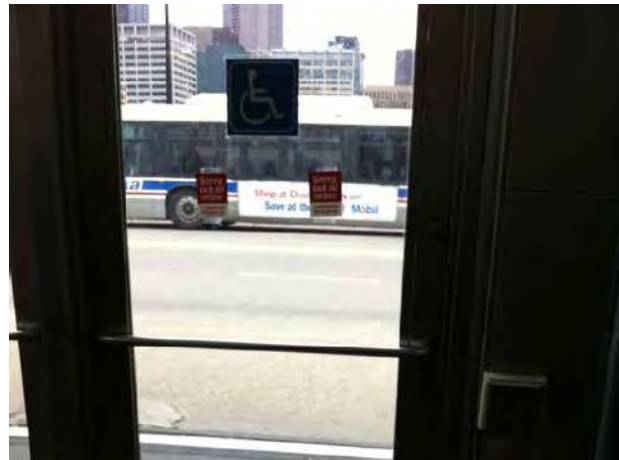
View of out of service ADA operator on Halsted stationhouse entry door
