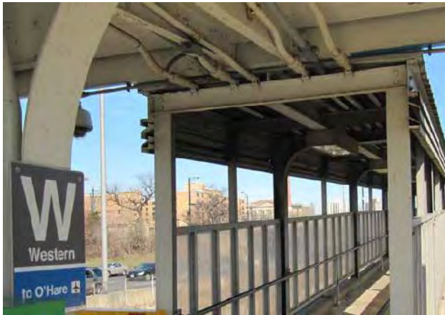
View of peeling paint and rusting conduit at platform canopy structure
