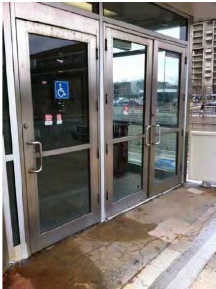
View of cracked concrete at entry door to Morgan stationhouse. Note that water is sitting on the concrete and that 2 out of 3 doors are out of service.
