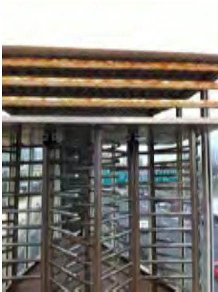
View of corrosion and deterioration at Peoria stationhouse exit only area
