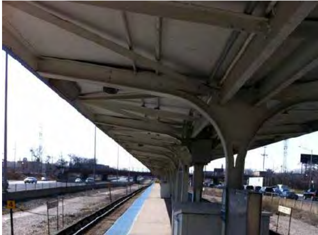
View of corrosion and peeling paint at underside of platform canopy
