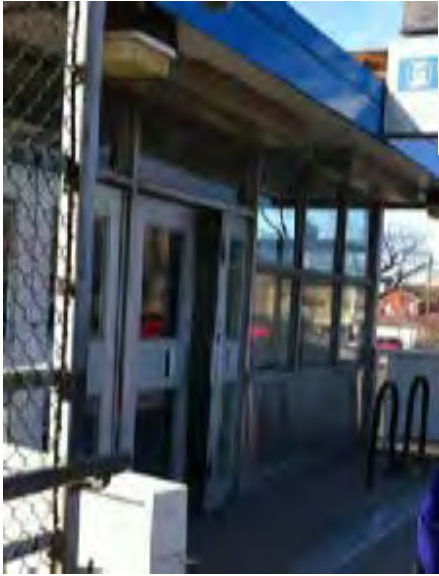
View of non-compliant doors at station house
