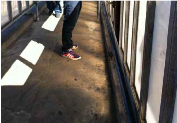
View of non-compliant ramp with no landings
