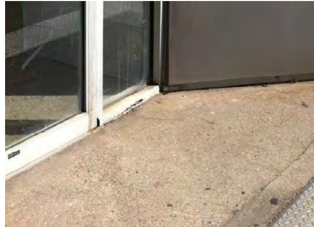
View of deterioration at the base of newer storefront at Damen stationhouse.
