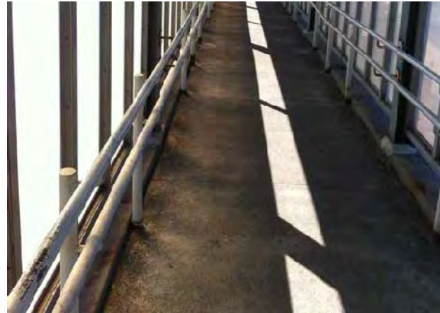
View of corrosion and rusting at posts of handrails on ramps. Note peeling paint on railings, and aged plastic panels on windbreaks.
