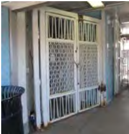
View of corrosion at gates in Loomis stationhouse
