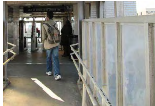
View of corroded surfaces and aged plastic panels of wind break enclosure at ramp
