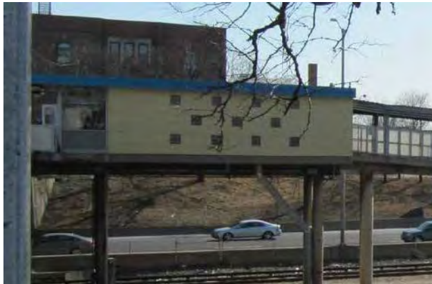
View of stationhouse exterior showing spalling at concrete at base of the wall
