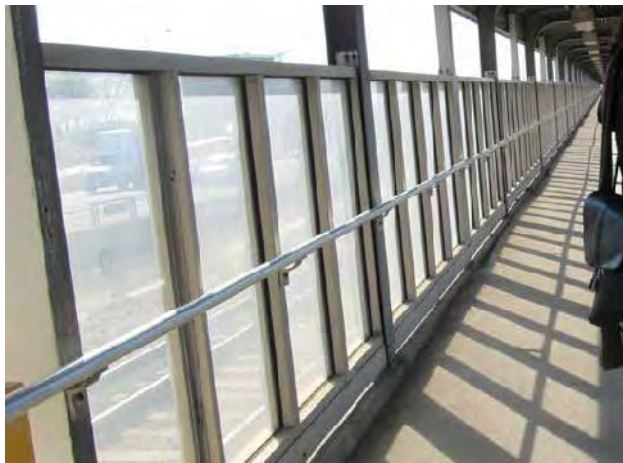
View of corrosion and scratched wind break panels at ramp.
