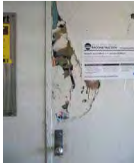
View layers of peeling paint in Loomis stationhouse
