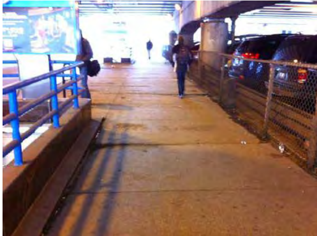
View of cracked and unlevel sidewalk at Clinton Street
