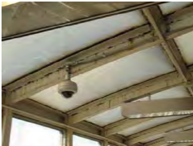
View of corrosion and deterioration at Peoria stationhouse skylight system
