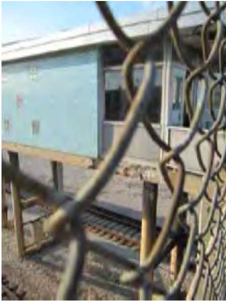
View of spalling concrete at the Racine stationhouse
