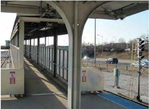
View of non-compliant ramp from platform to station house
