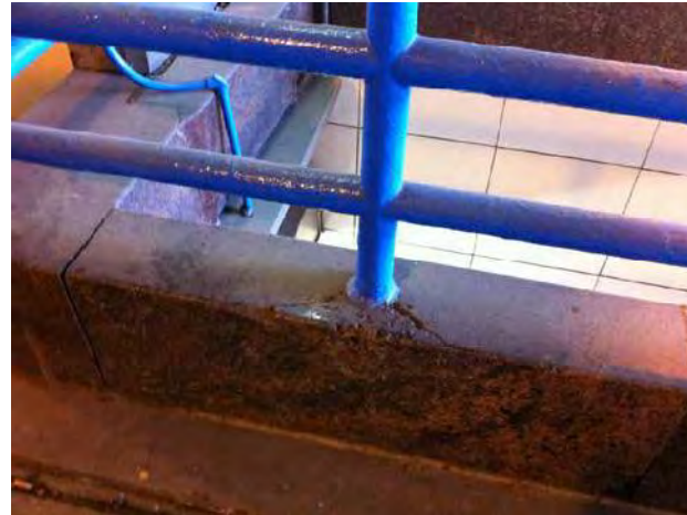
View of cracked stone cap at stair railing
