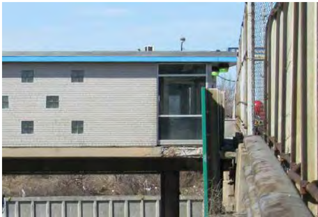
View of spalling concrete at base of Kedzie Stationhouse walls, rusting and loose concrete is evident.
