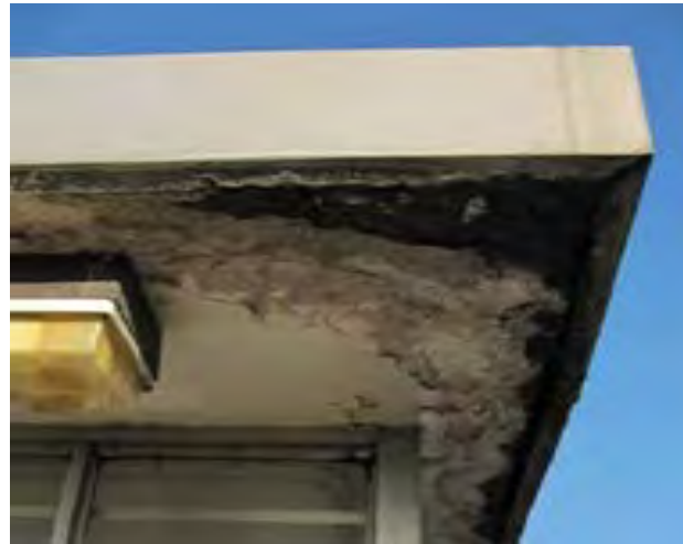
View extensive water damage at Loomis stationhouse roof eave
