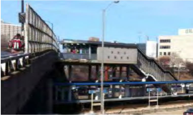
View of corrosion and deterioration at concrete base at Ogden stationhouse
