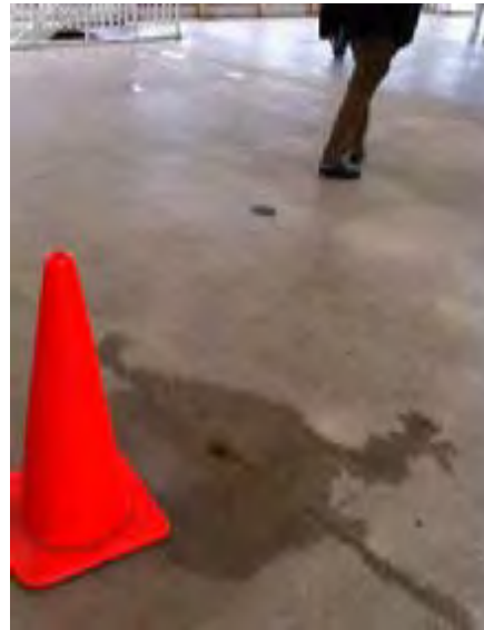
View of evidence of roof leaks at Peoria stationhouse skylight system
