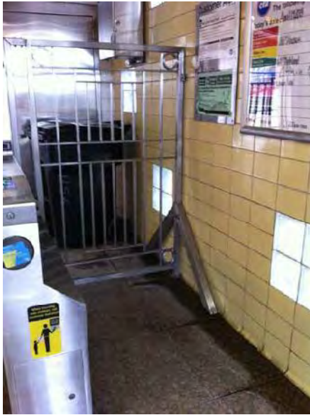
View of water infiltration in Morgan stationhouse
