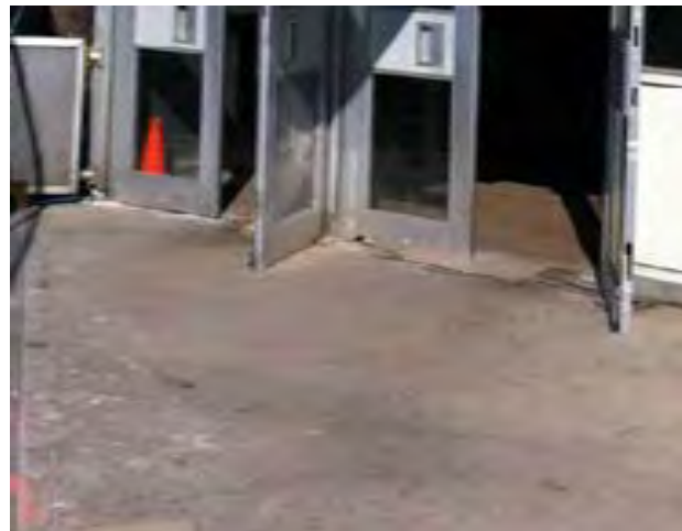
View of deterioration at the base of doors and storefront at Ogden stationhouse.
