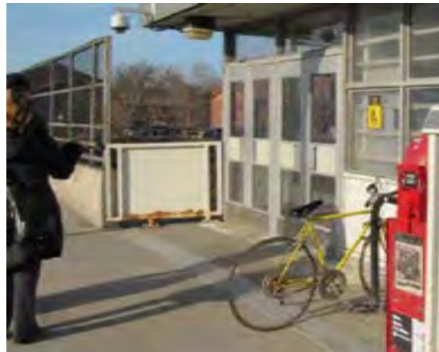
View of non-compliant entry doors at Loomis Street Stationhouse
