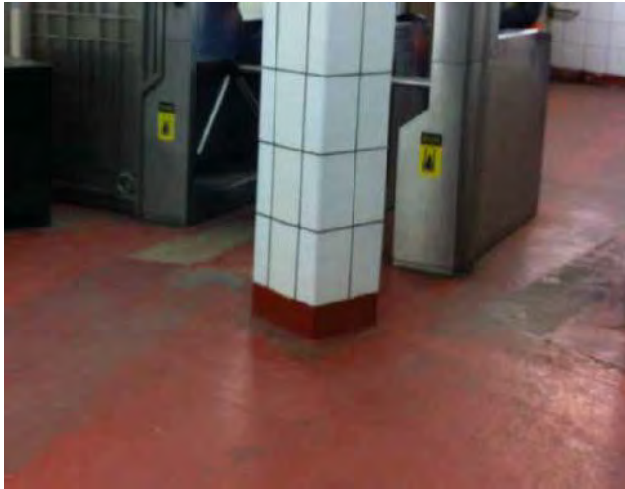
View of cracked and patched floor in station paid area
