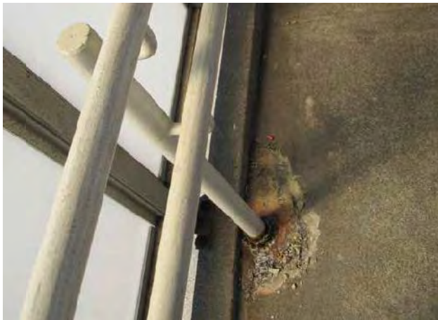
View of corrosion, rusting and deterioration at base of handrail supports in Morgan stationhouse ramp
