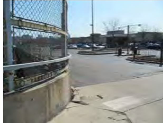
View of non-compliant curb ramp at Congress Parkway on approach to Morgan stationhouse. Note that the pedestrian crosswalk is not identified with striping
