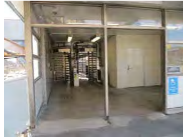
View of non-compliant entry at Paulina Stationhouse
