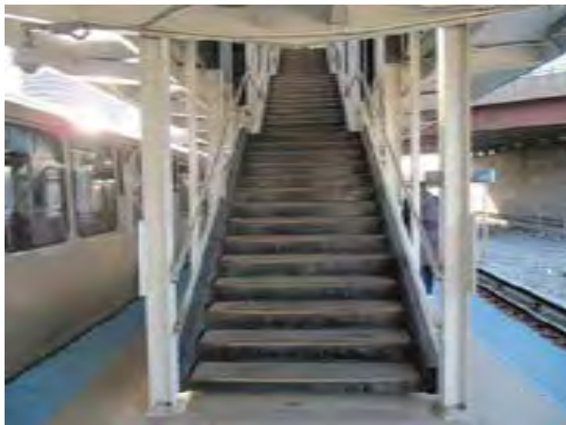
View of non-compliant platform with impeding stair element
