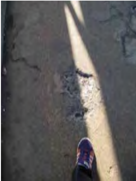
View of broken and cracked walking surface of ramp
