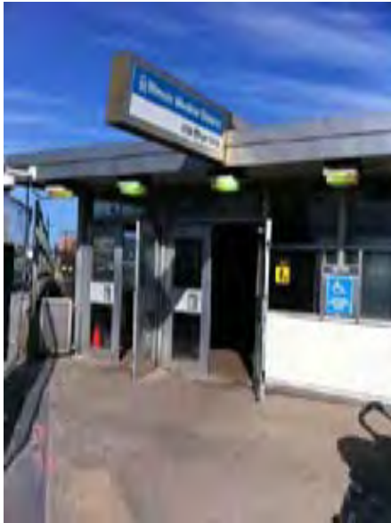
View of non-compliant entry doors at Ogden Stationhouse
