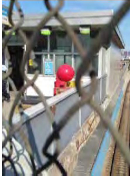
View of corrosion and deterioration at concrete base at Ogden stationhouse
