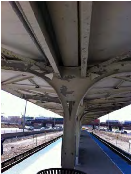
View of peeling paint and rusting conduit at platform canopy structure
