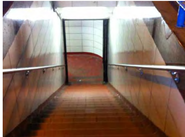
View of cracked and patch surface of entry stairs
