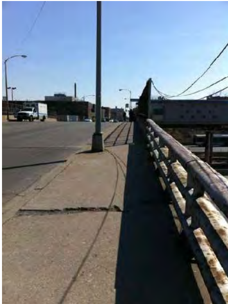
View of sidewalk along Kedzie Avenue on approach to station. Note cracked concrete sidewalk that should be repaired.
