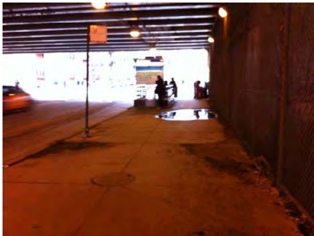
View of cracked and uneven sidewalks on approach along the west side of Clinton Street
