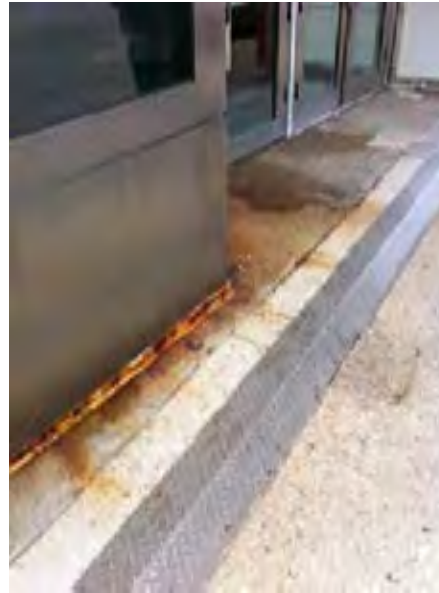
View of rusting and staining at base of customer service kiosk at Morgan stationhouse entry
