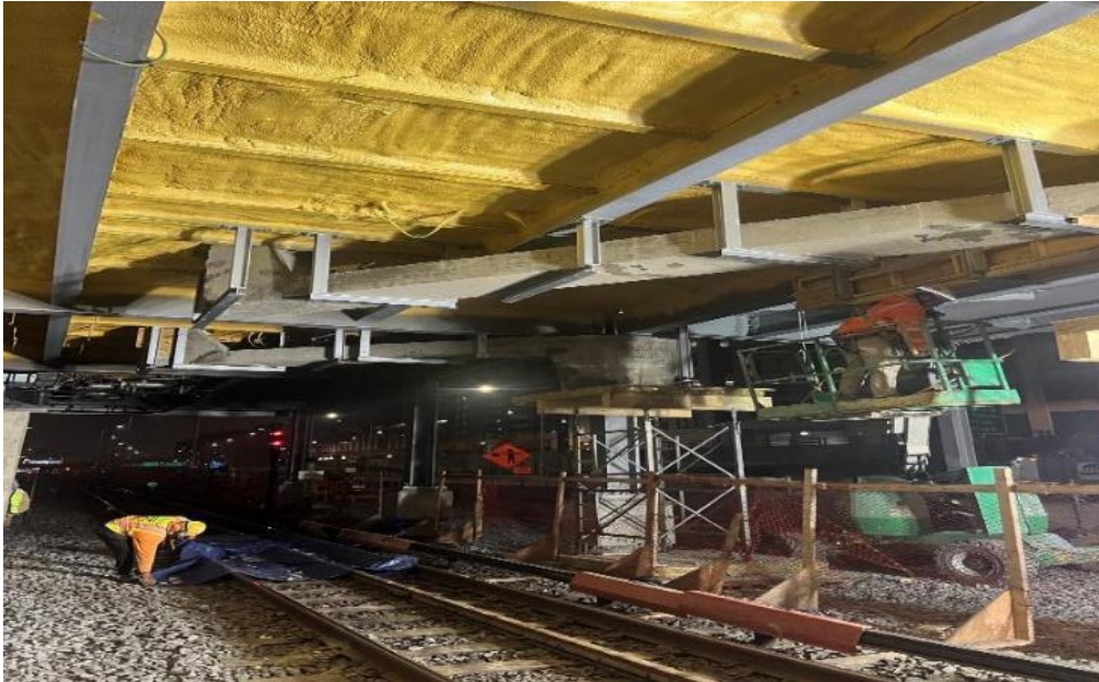
Concrete Suspended Ductbank at Morgan Substation
