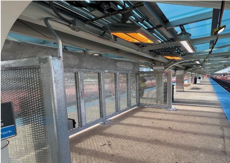
Racine Platform Windbreak and Infrared Heaters
