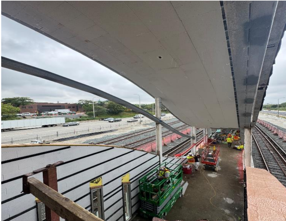
Racine Stationhouse Stairway Ceiling
