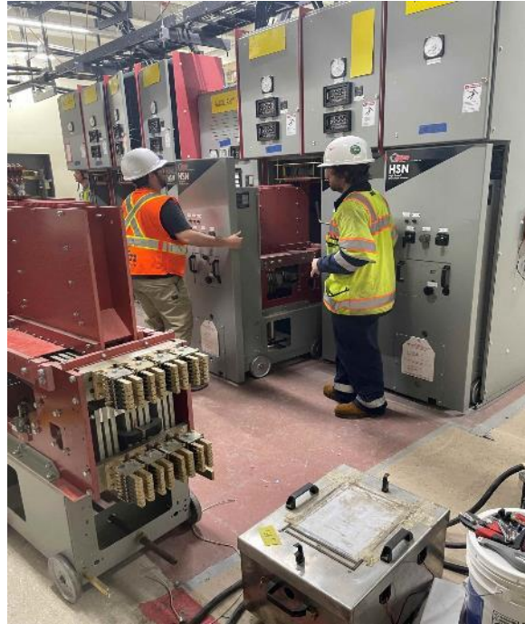
Barry Switchgear Testing
