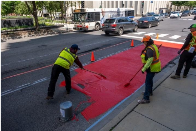
CDOT crews shown painting a portion of the street surface red to demarcate a new stretch of bus only lane along Chicago Avenue. Work is part of ongoing efforts by CTA and CDOT to prioritize bus services along congested corridors.
