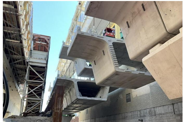
Pre-cast segments hang in place before being permanently sealed together to make a portion of the new elevated structure being constructed as part of RPM Phase One work.
