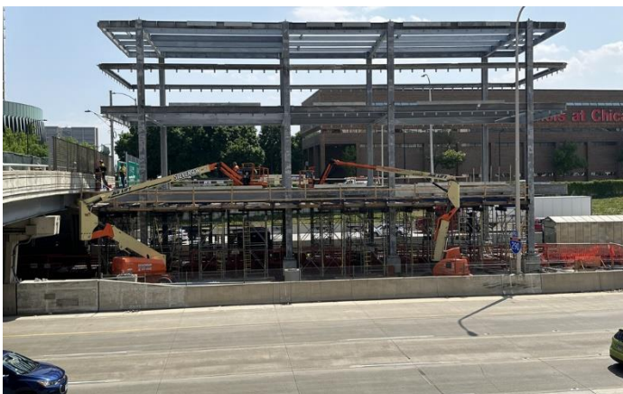
Crews constructing the new main stationhouse of the Racine Blue Line stop this spring.
