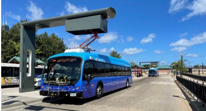
A CTA electric bus charges using the high-powered, overhead charger at the Navy Pier bus-turnaround.
