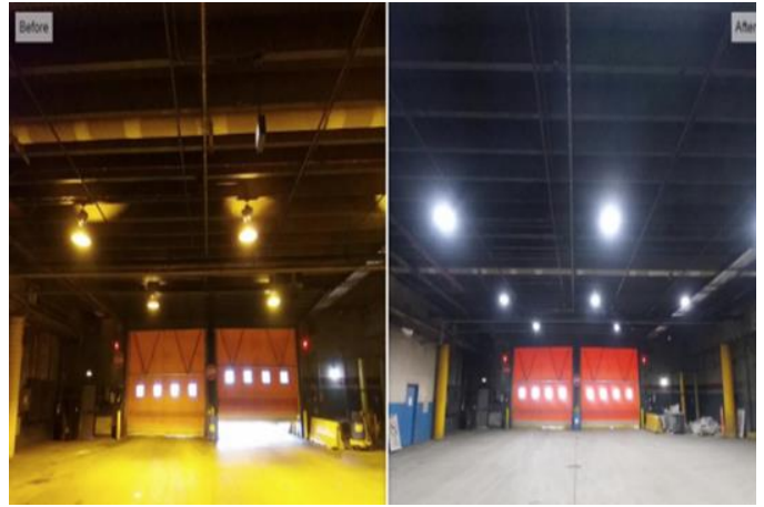
Lighting upgrades in bus garages and rail shops, along with more fuel-efficient buses, reduce regional emissions with cost savings of $3 million per year.
