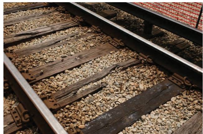
Continued capital investments and funding is critical to allowing CTA to replace worn out track and infrastructure that is beyond its useful life and in need of replacement. Shown is a stretch of track where trains were once limited to operating at 15 m.p.h.
