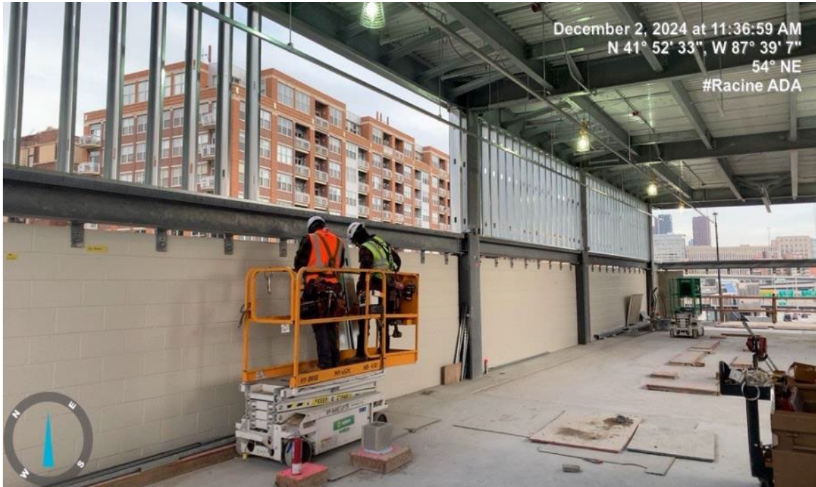
Morgan Substation 2 nd Level Louvers
