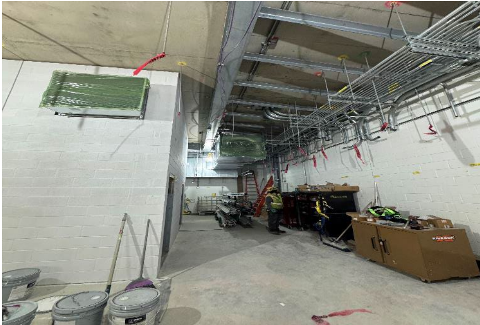
Morgan Substation 1st Level Conduits and Bus Duct
