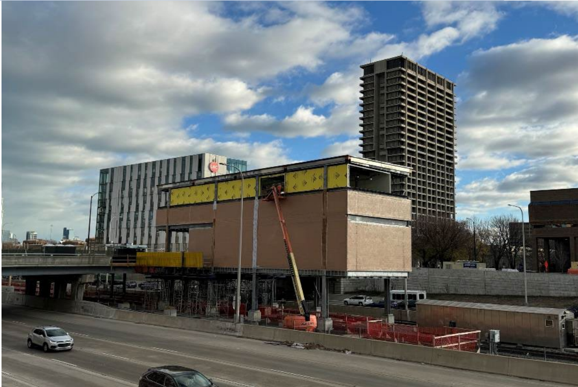
Morgan Substation Looking SE
