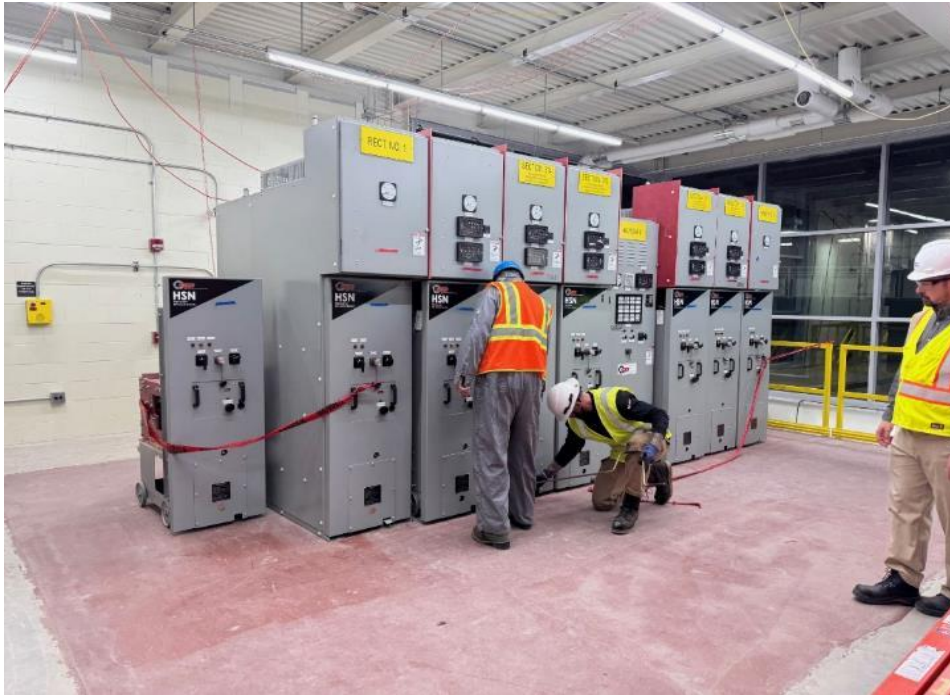
Short Circuit Testing at Damen
