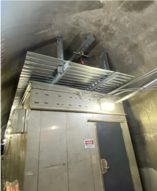
Completed Drip Pan at Canal Tie-House
