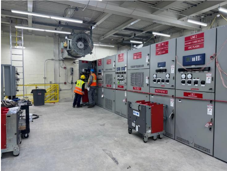
Short Circuit Testing at Damen
