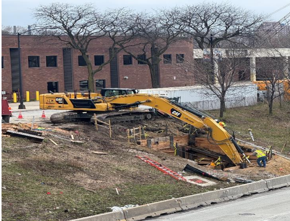
Racine Electrical Receiving Pit
