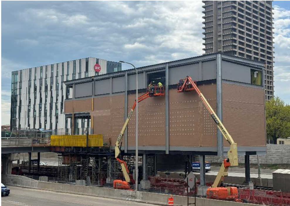
Morgan Substation Looking Southeast
