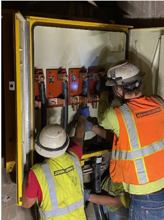
Barry Subway Cable Landing
