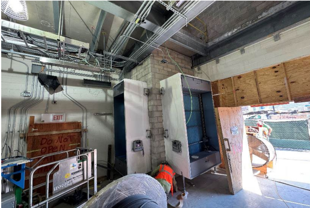
Morgan Substation HVAC Intake Insulation
