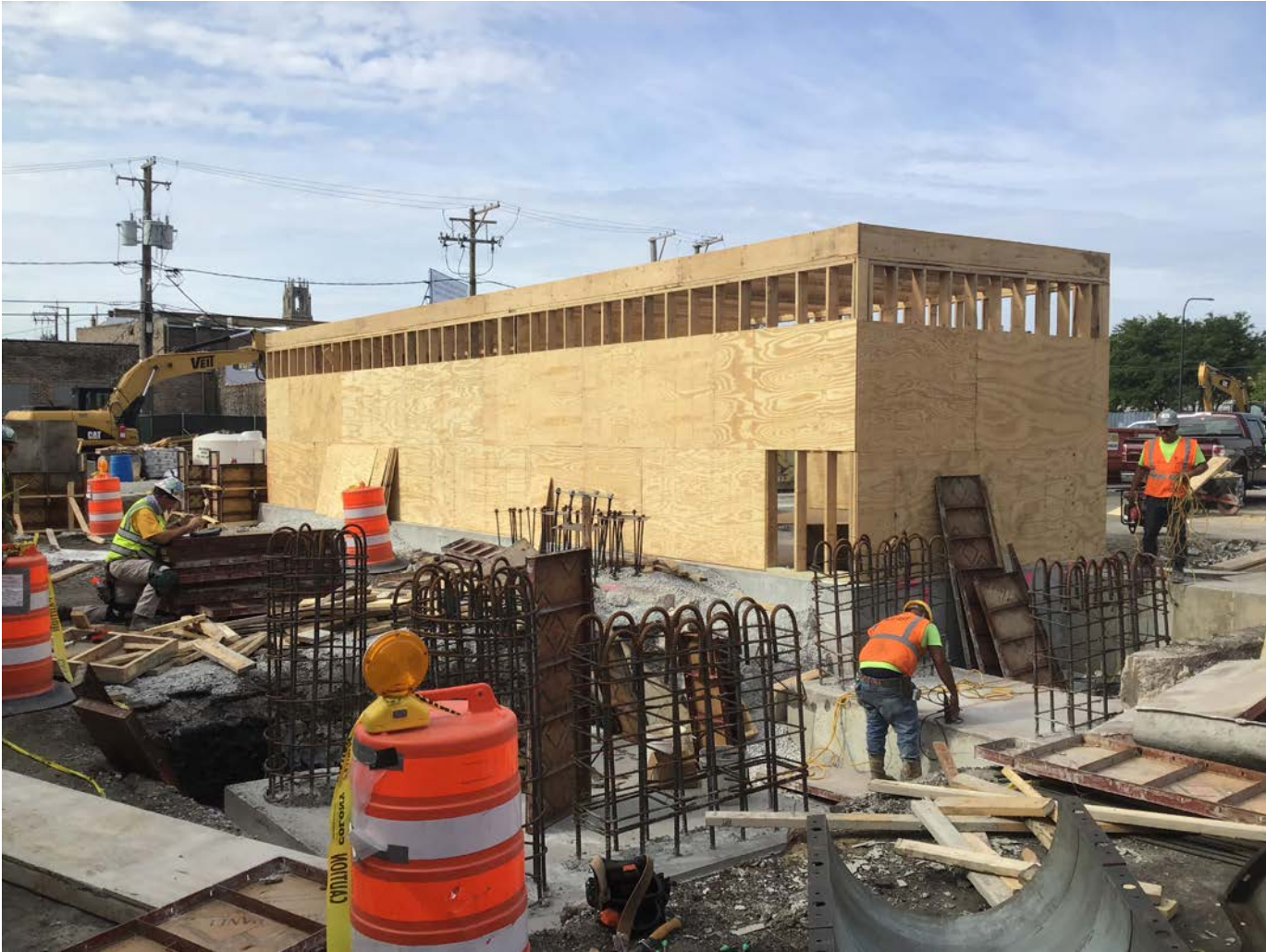
Lawrence to Bryn Mawr Modernization – Support Rooms and Foundations at Bryn Mawr Temp Station
