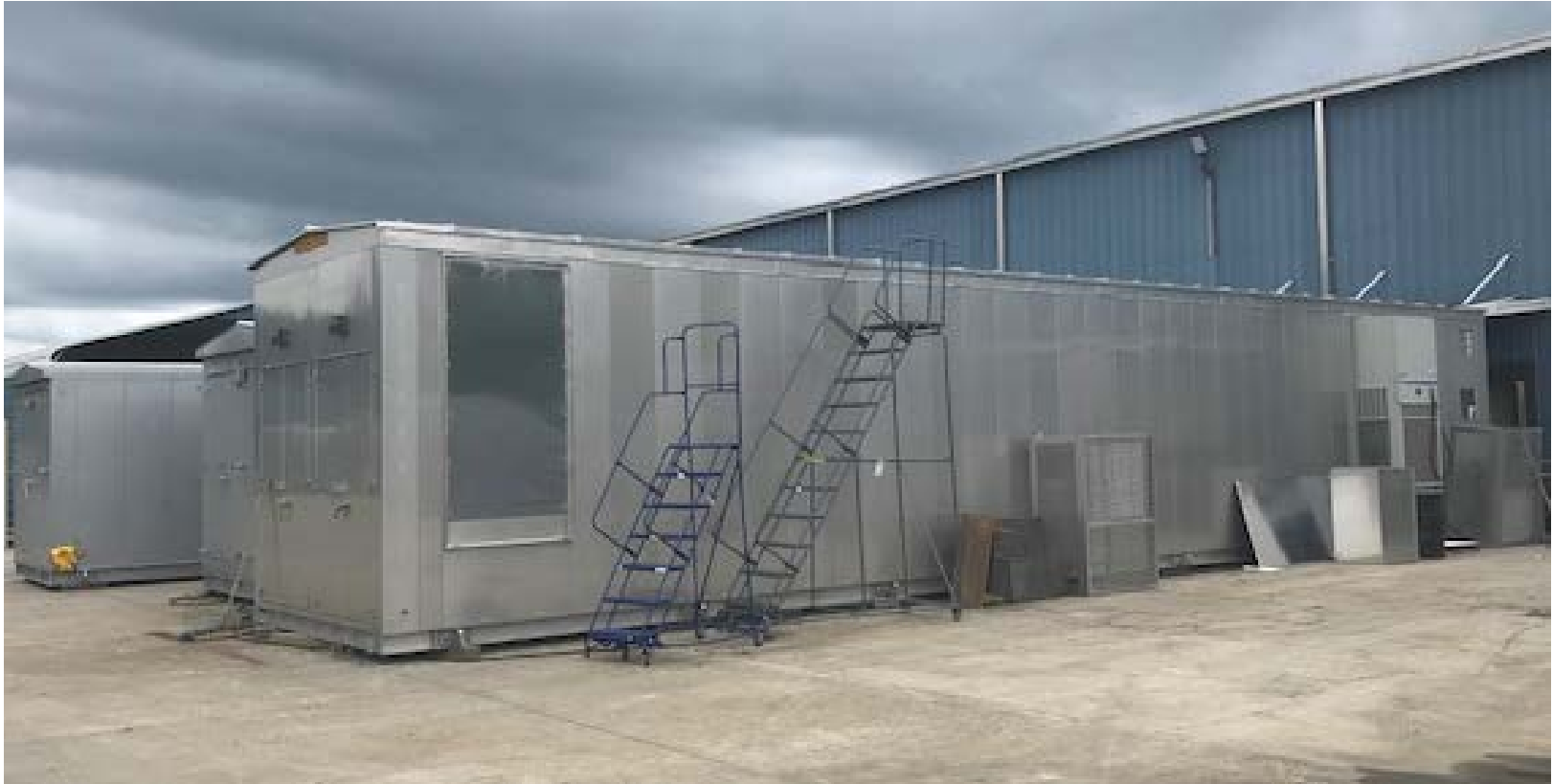
Lawrence to Bryn Mawr Modernization – Montrose Relay House prior to Shipping
